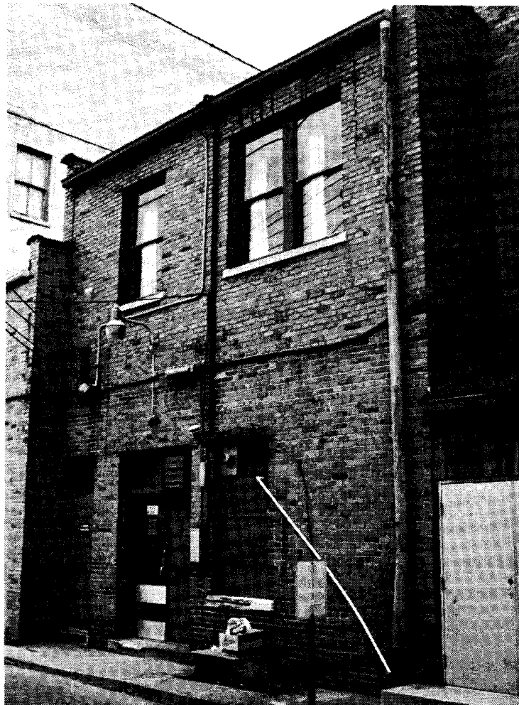
This Barberton commercial building has a very simple roof, gutter, and downspout system that is easy to install and maintain. It is important that gutters and downspouts be properly sized to carry away the water typically shed by the roof.
