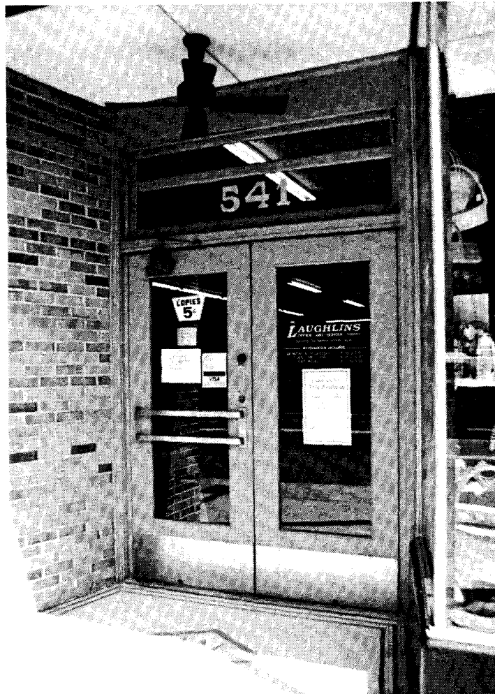
These paired doors with a transom above are typical of commercial buildings from the late 19th and early 20th centuries. Note the simplicity of the overall design of the entrance. The recessed doors provided weather protection.
